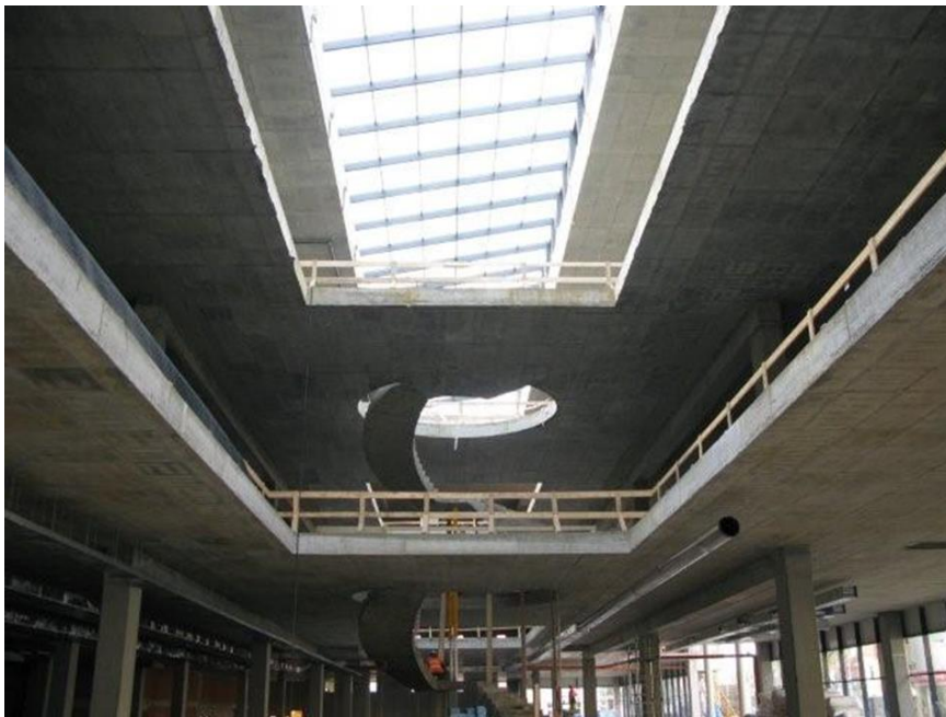
Figure 5.9. large opening made into Contruss floor
