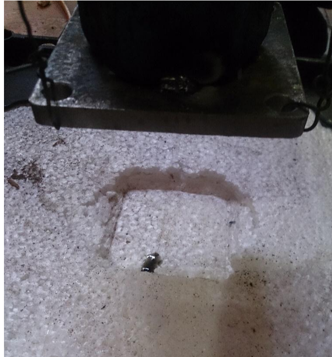
Figure 5. localized deformation under location of load
