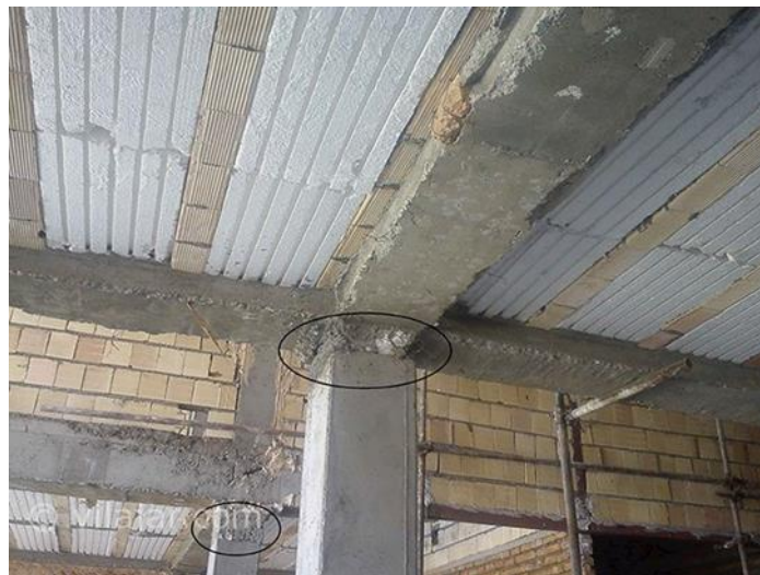
Figure 2.3. Honeycombing in concrete in the connection of column and diaphragm
